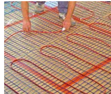
Heating cables connection.
