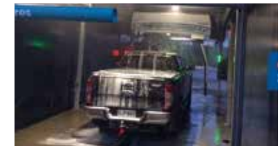
Connection of LED luminaires in a car washing plant (New Zealand). Series TH387.
